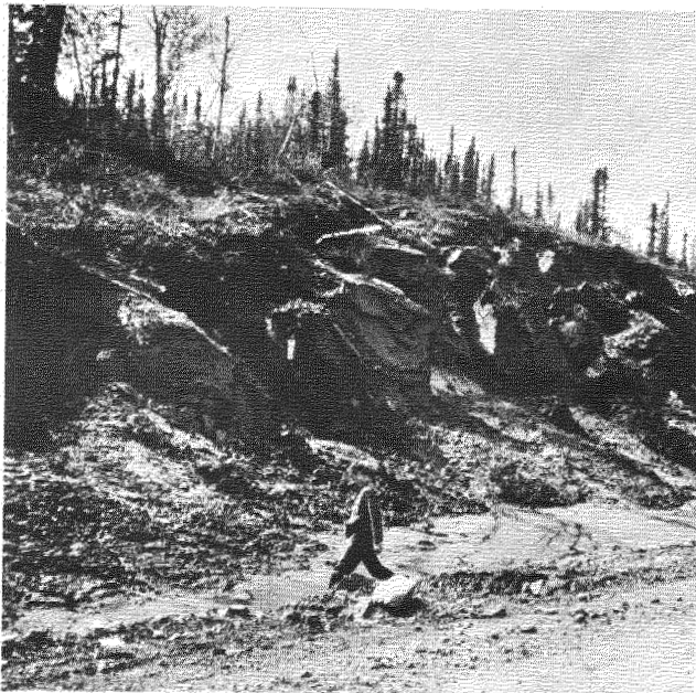
FIGURE 4 Thawing backslope, 31.6 km, 26 June 1970.
