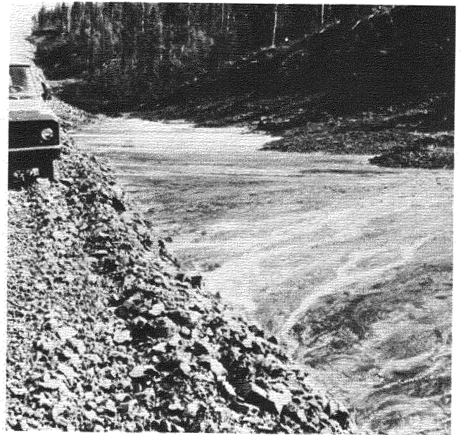
FIGURE 5 Backslope erosion into parallel ditch, 31.6 km, 26 June 1970.
