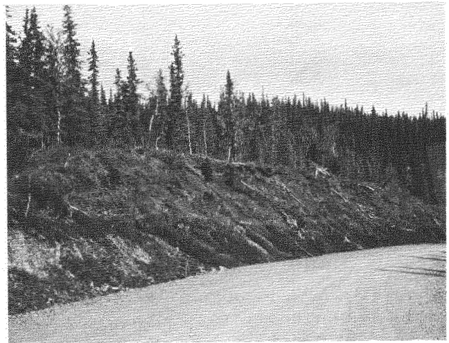
FIGURE 16 More stable backslope, 32.6 km, 17 August 1971.
