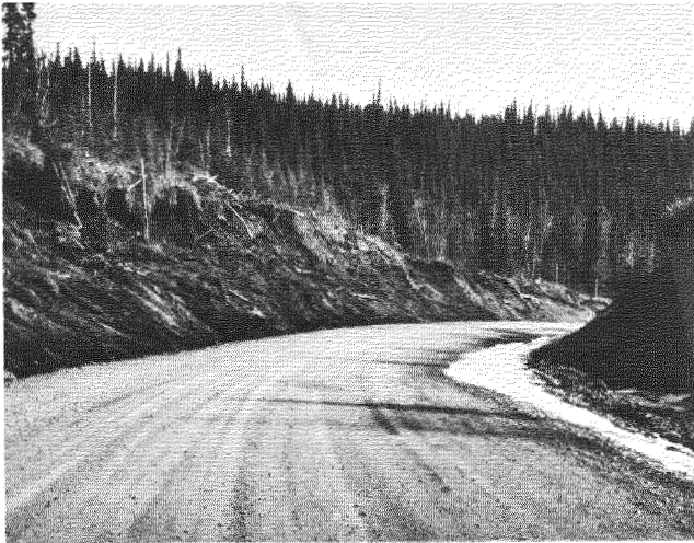
FIGURE 14 Additional slumping of backslope, 32.6 km, 28 May 1971.
