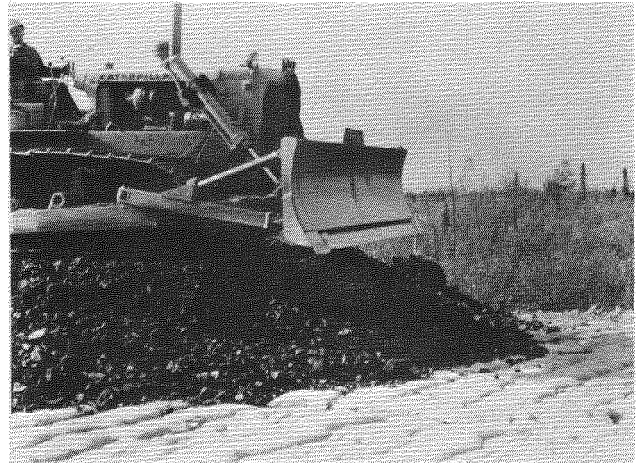
Figure 2. End-dumping the topping gravel lift. Rocks 0.3-0.6 m across produced only minor scuff marks on the foam surface, while the weight of the bulldozer and gravel layer did not damage the foam.
