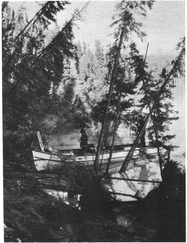
Figure 5: Slumping of undercut clay bank at Site 2 with fallen trees along the foreshore.
