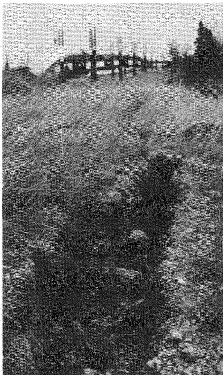
PLATE 2 Ground crack at MP 393
