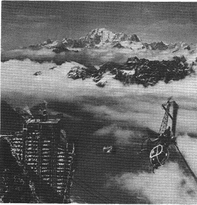
Figure 5: Concrete transportation to the construction site of the summit station at 3,820 m a.s.l. Concrete was prepared at "Trockener Steg" to avoid frost problems. Mont Blanc (French Alps), the highest peak of the Alps, is visible in the background. (Photograph taken by Air Zermatt.)
