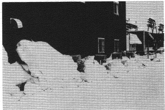
FIGURE 7 Exhaust Ducts Note drifting snow.
