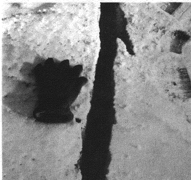
Fig. 4 A large thermal contraction crack formed the first winter at Illisarvik.
