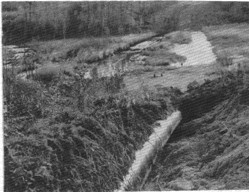
Figure 1. The first part of the gas pipe-line Mastakh-Yakutsk on the swampy site.
