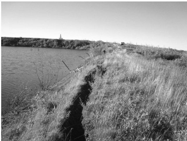
Figure 8. Vortac Dam site photograph with visible upslope active slumping (September 9, 2010). FAA Vortac structure visible in background.
