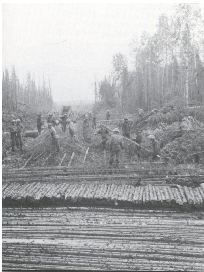
Figure 3. Corduroy road construction used to mitigate damage to the pioneer road caused by thaw of ice-rich permafrost. Timbers were obtained from slash created by road construction and covered with brush and gravel to inhibit thaw. Three of the seven U.S. Army regiments (93 rd , 95 th , 97 th ) involved in construction of the pioneer road were composed of African-American troops (Twichell 1992, Brinkley 2002).
