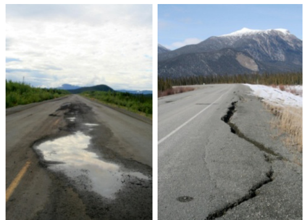
Figure 2. Left: thaw-settlements causing water to pond in the depression near the centerline of the road (km 1858). Right: longitudinal cracking observed along the Alaska Highway (km 1760).
