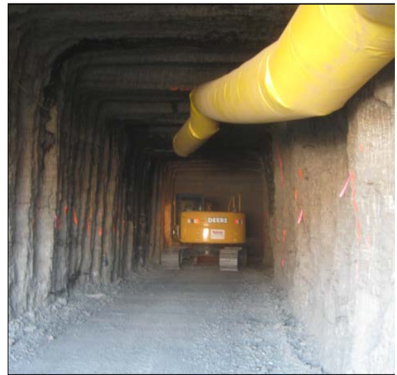
Figure 6. View of the New Tunnel. At the time of this photo, the face was at a horizontal depth of 26.3 m.
