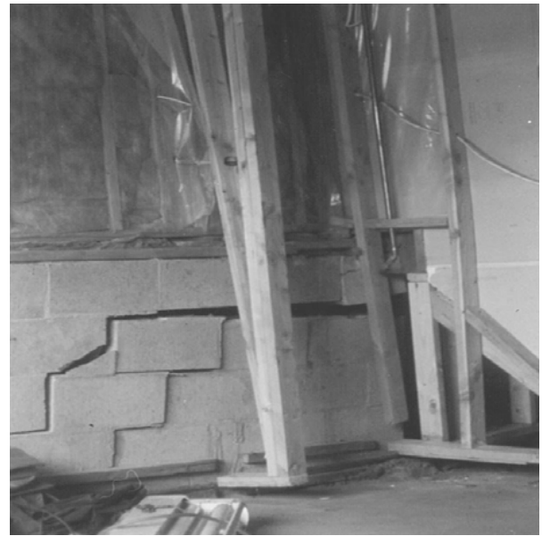
Figure 3a. Interior wall damage at a house located on Knights Way (Castle Heights Subdivision).
