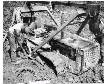
Figure 2. Small bulldozer mired in mud after thaw of ice-rich permafrost.
