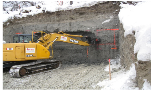
Figure 3. EC-25 mounted on the boom of a 13-t excavator for the Phase I excavation.
