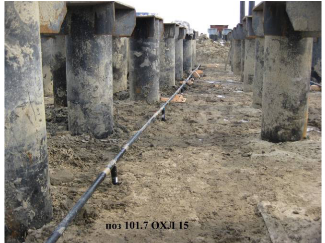
Figure 6. Foundation soil thermal stabilization with the VNP system at a production building in the Bovanenkovo Gas Condensate Field.
