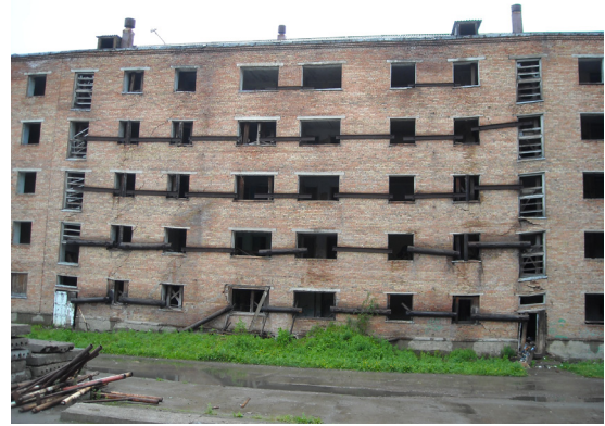
Figure 7. Deformation in the first housing estate of Igarka (July 2010) due to the reduction of bearing capacity of the permafrost piles.
