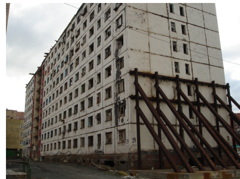
Figure 8. Housing at Laureatov Street in Norilsk. Irregular settlement of permafrost piles due to the warming and partial thawing of the surrounding permafrost, August 2009.
