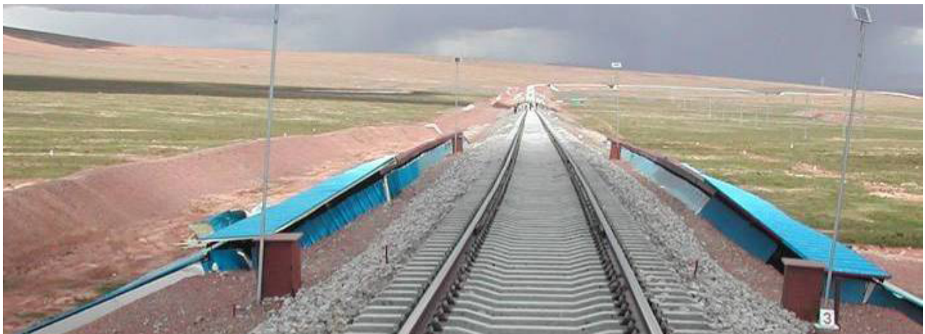
Figure 5. Sun and precipitation awnings on the Qinghai-Tibet Railway at the site of ice-rich ground in the subgrade, August 2006.
