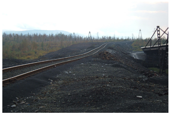
Figure 2. Long-wave longitudinal deformation of the rail roadbed near the Valek crossing loop. Length of wave \approx 120 m.
