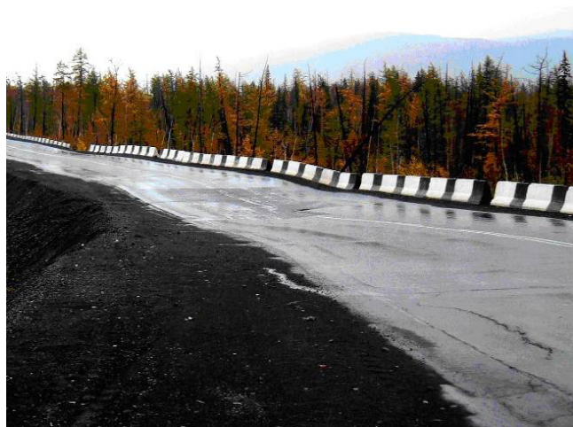
Figure 4. Local subsidence formation on the Norilsk-Talnakh auto road.
