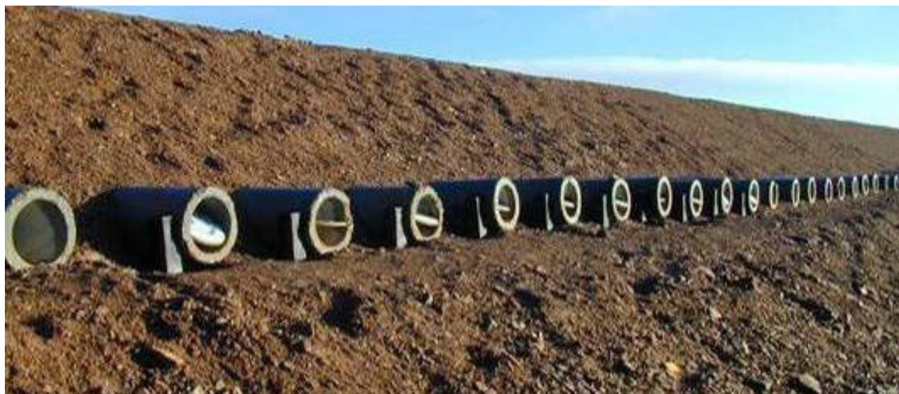
Figure 7. Transversal ventilated reinforced concrete pipes in the roadbed of the Qinghai-Tibet Railway (photograph by Niu Fujin).
