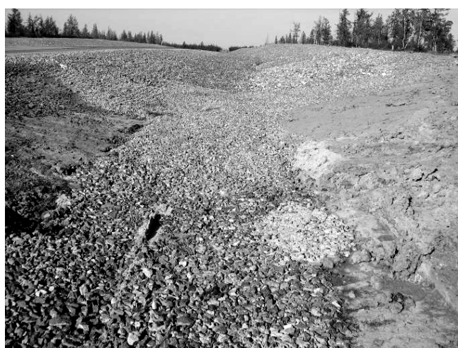
Figure 2. Erosion-control structure with a geogrid filled with crushed stone. Photo taken in 2010.
