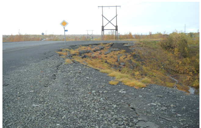
Figure 7. Stepwise settlement of the main embankment site of the Norilsk-Talnakh auto road.
