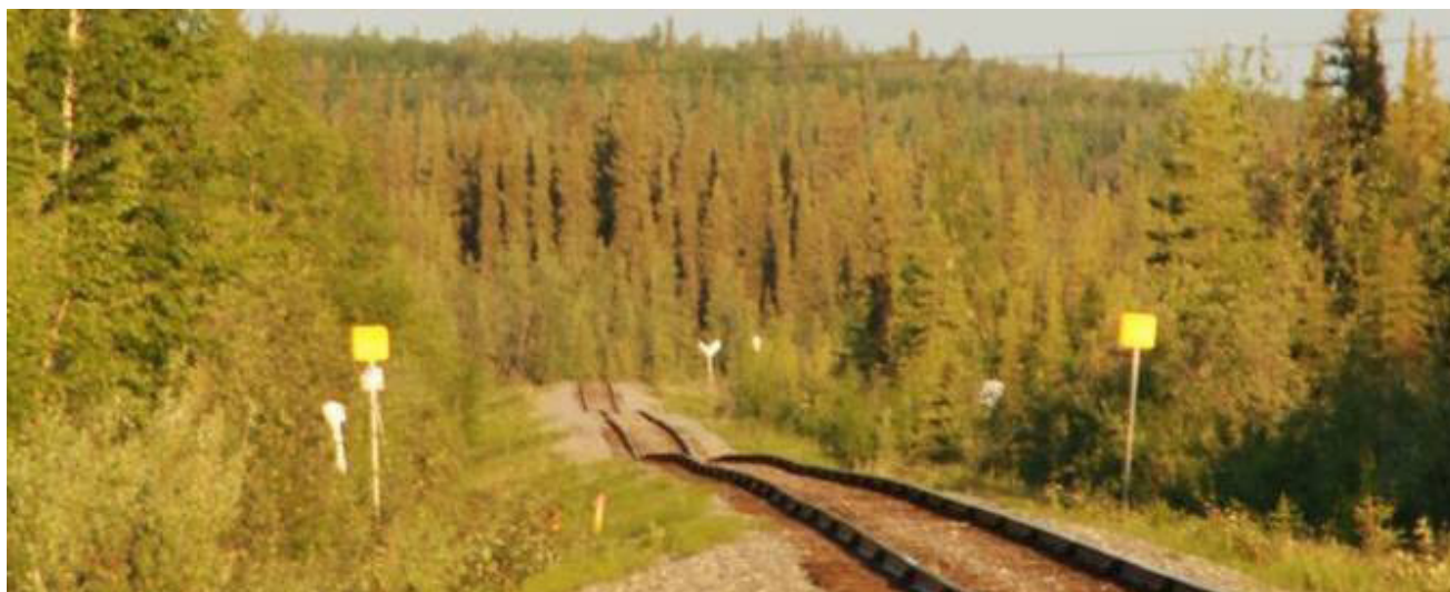
Figure 3. Alaska Railroad track deformation near Fairbanks, July 2008.
