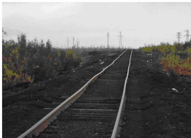
Figure 5. Nature of deformations on the low embankment zone.
