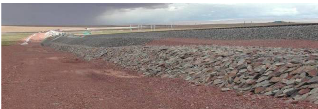
Figure 4. Qinghai-Tibet Railway track deformation, August 2006.
