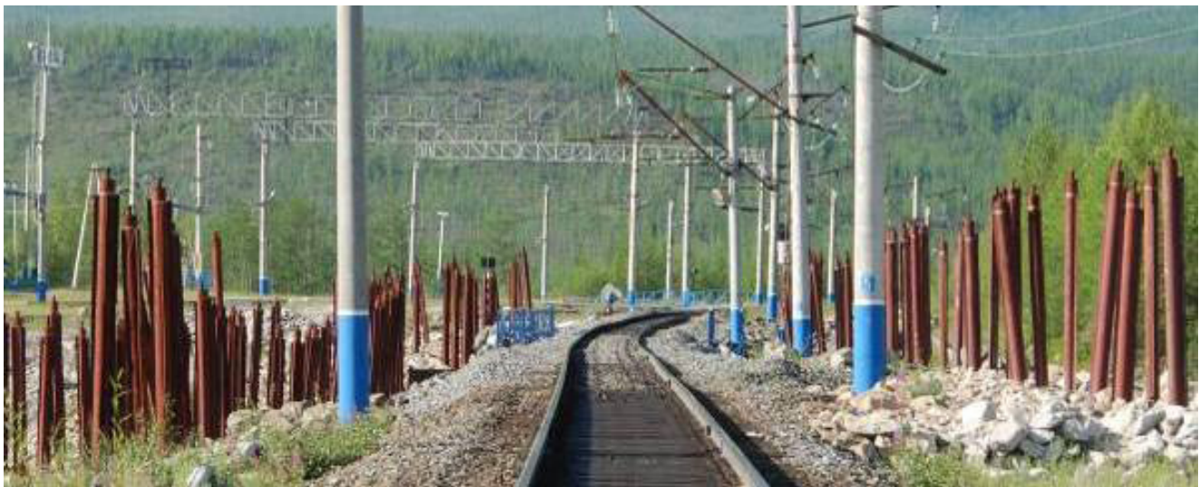
Figure 2. East-Siberian Railway track deformation, 1374 km of the Baikal-Amur Railway (BAM), July 2011.
