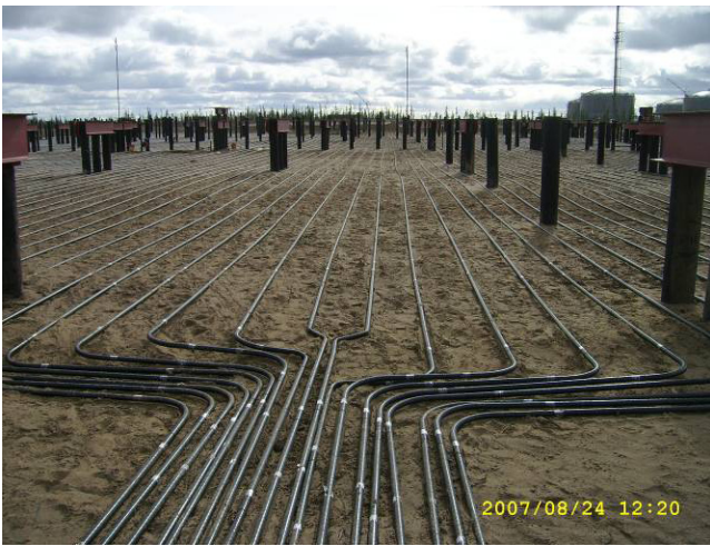
Figure 4. Foundation soil thermal stabilization using the HNP system at a production building (116.2 x 66 m) in the Vankor Oil Field.
