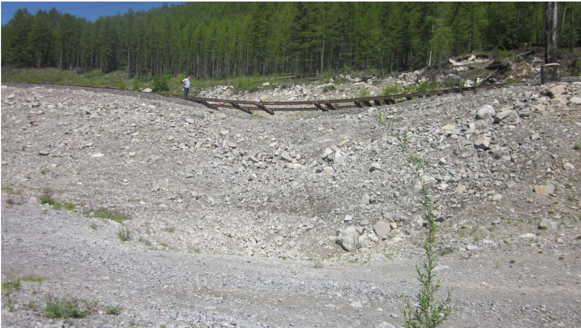
Photo 4. Abandoned Chena-Chara Railway. July, 2012 view of segment exhibiting significant thaw settlement since closure in 2002.
