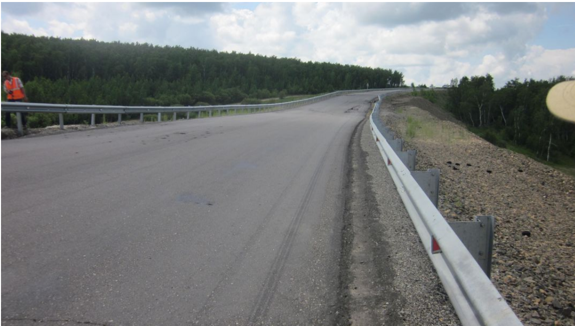
Photo 2. Trans Siberian Highway (Route 55). July, 2012 view of continuing major embankment failure resulting from underlying foundation permafrost degradation.
